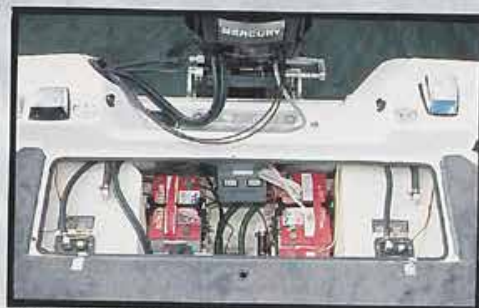
Fuel Tanks & Battery Area
