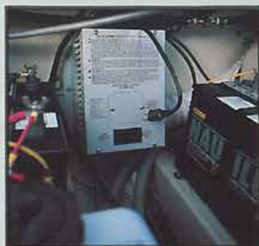
Dual Built-In Custom Lester Battery Chargers
