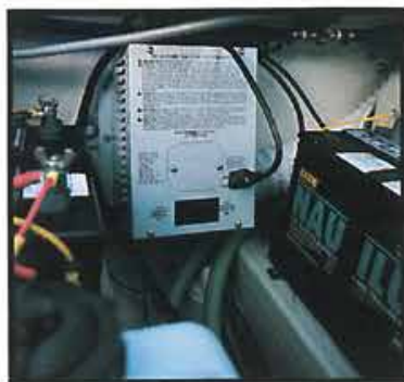
Built-In Custom Lester Battery Chargers (3)
